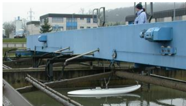
Figure 3: Float with FVP sensor below the scraper bridge in a CSO tank in Pétange (Luxembourg)
