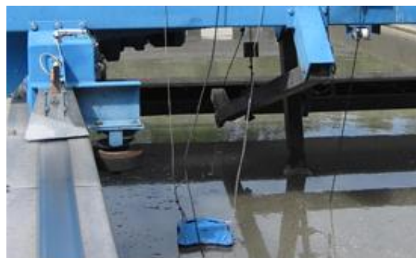
Figure 4: Float with FVP sensor below the scraper bridge in a primary clarifier in Pétange (Luxembourg)
